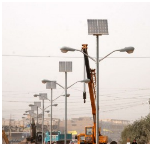
Solar panels power more than 1,200 street lights, providing illumination for more than 35 kilometers of roadway in and around Fallujah, Iraq. Photo courtesy of the U.S. Army Corps of Engineers
